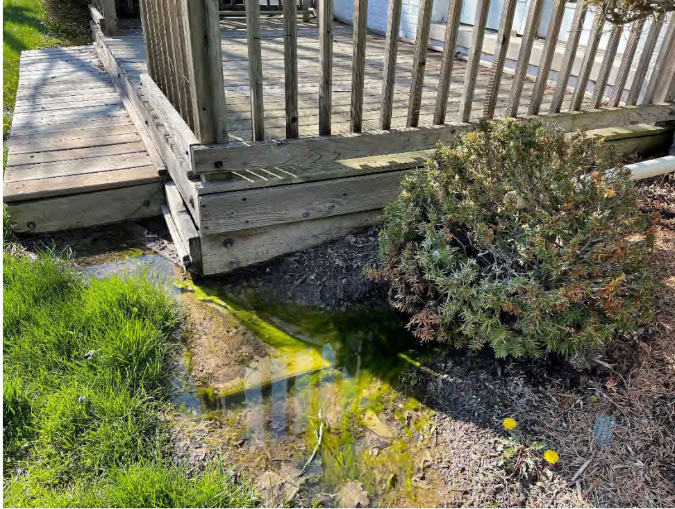
5. Sump pump outlet showing ponded conditions near deck on south side of residence.
